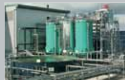
Avlon Wastewater Treatment Plant /22
